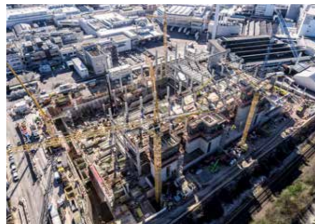
Where the future has tradition: The assembly building for the first electric Porsche vehicles is being constructed in Plant 2.
